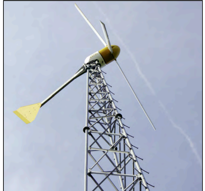
Mike Mills’ wind turbine has garnered interest from curious passers-by. The turbine generates enough electricity to take care of two-thirds of Mills’ household power needs.
