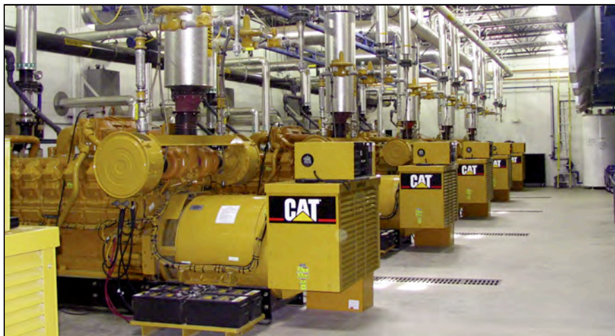
(top) The Two Pine Landfill accepts waste from Jacksonville, Sherwood, Cabot, Conway, rural Pulaski County and as far away as Garland County. (bottom) Six engines convert 500,000 tons of waste annually into electricity for North Little Rock residents.
